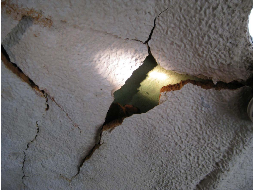
Picture 20: Ceiling Damage 2
