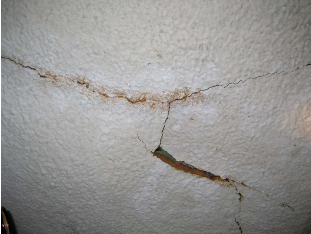
Picture 21: Ceiling Damage 3
