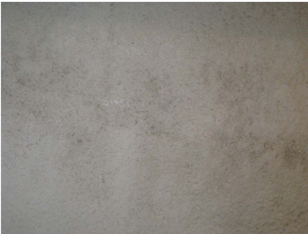
Picture 11: Mold, Bathroom Wall
