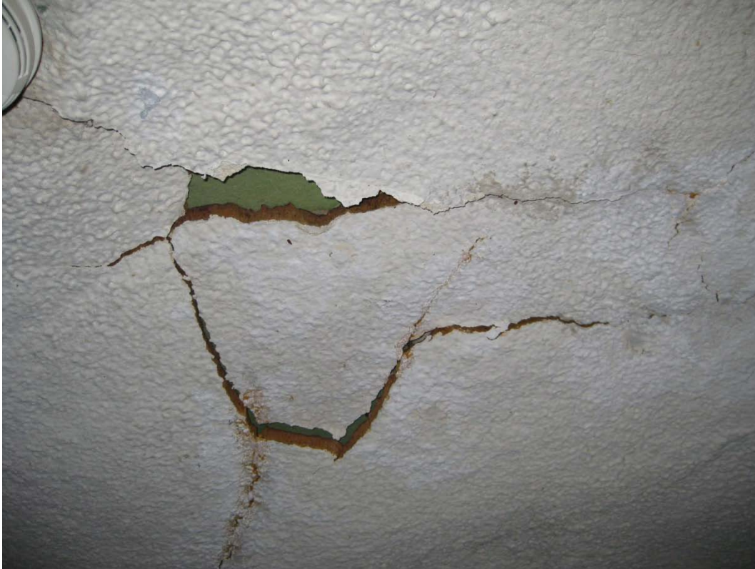
Picture 19: Ceiling Damage 1
