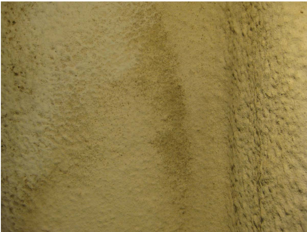
Picture 13: Mold, Bathroom Walls
