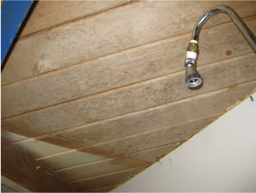
Picture 12: Mold, Bathroom Ceiling
