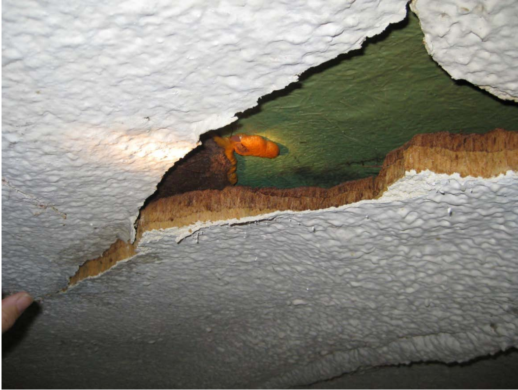
Picture 22: Ceiling Damage 4
