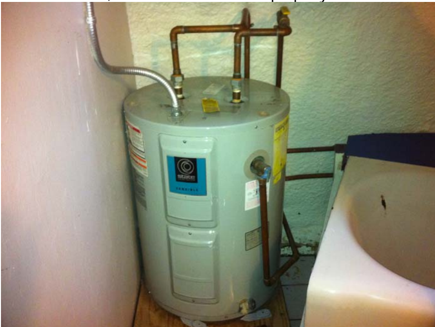
M-2: Dome #4, water heater tank not properly braced.
