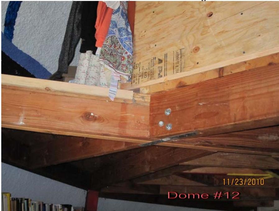
S-3: Dome #12, Condition B, Intersection of girders.
