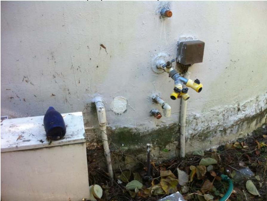
M-4: Dome #12, improper backflow prevention device.
