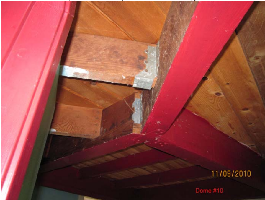
S-2: Dome #10, Condition B, Intersection of girders.
