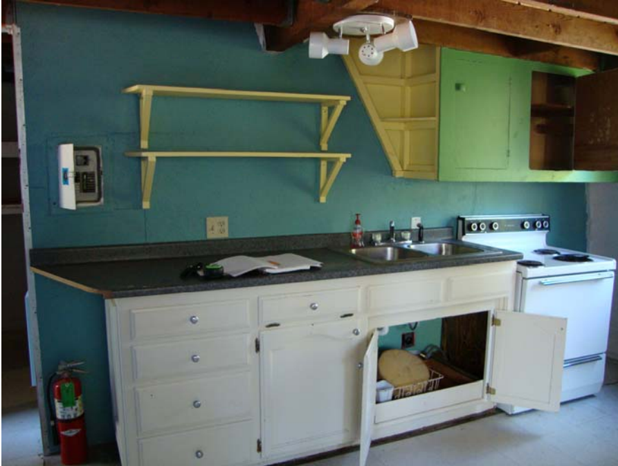
M-1: Dome #10, combustible material above cooking range.
