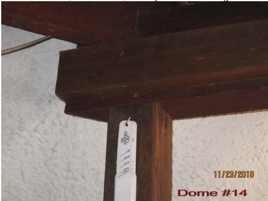
S-4: Dome #14, Condition C, inadequate column to girder connection
